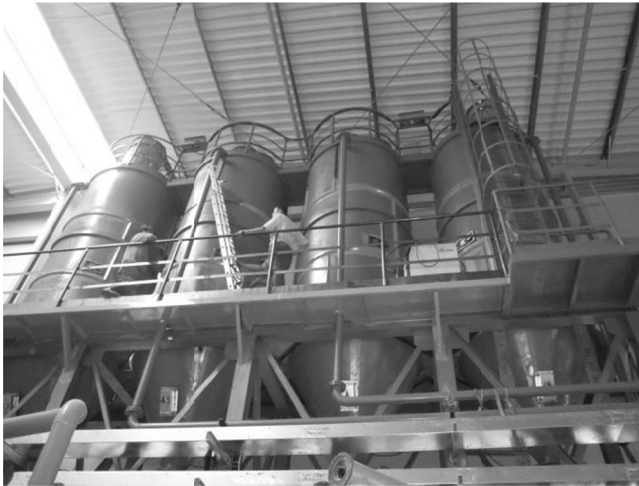
Fig 1-8. Sample daily stock silos, with a capacity of 15 \text{ m}^3 each.
