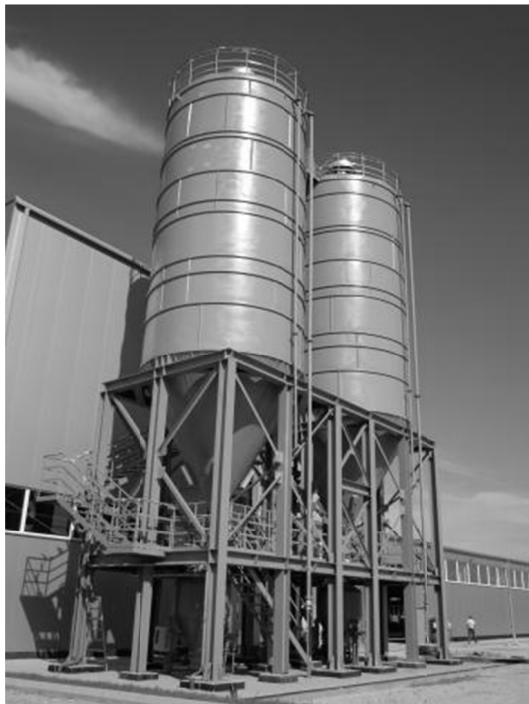
Fig. 1-6. Raw material silos, with a capacity of 200 m 3 each, outside the shop floor.
