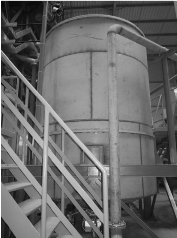
Fig. 1-10. Sample water tank with a capacity of 25 m 3 .
