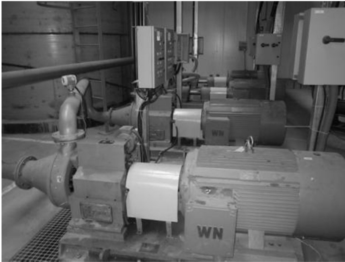
Fig. 1-13. View of four refiners.
