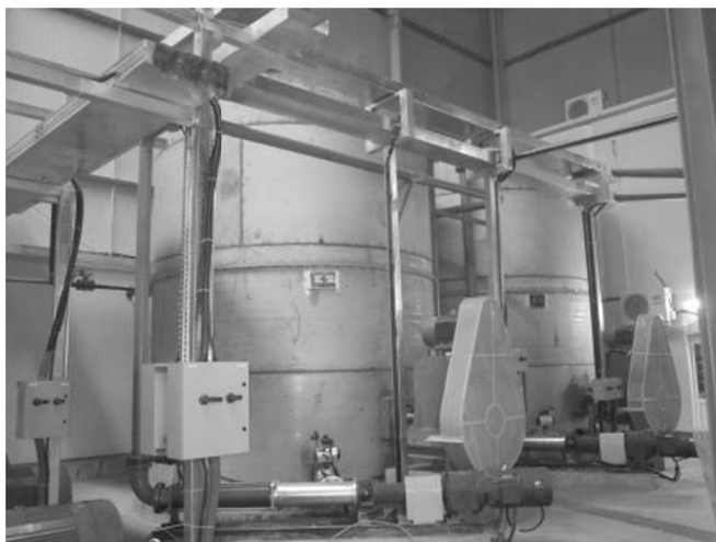
Fig. 1-14. Refined pulp storage tanks with capacity of 50 \text{ m}^3 .
