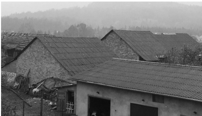
Fig. 1. Corrugated roofing made of asbestos FCB, now expected to be removed due to health risks.
